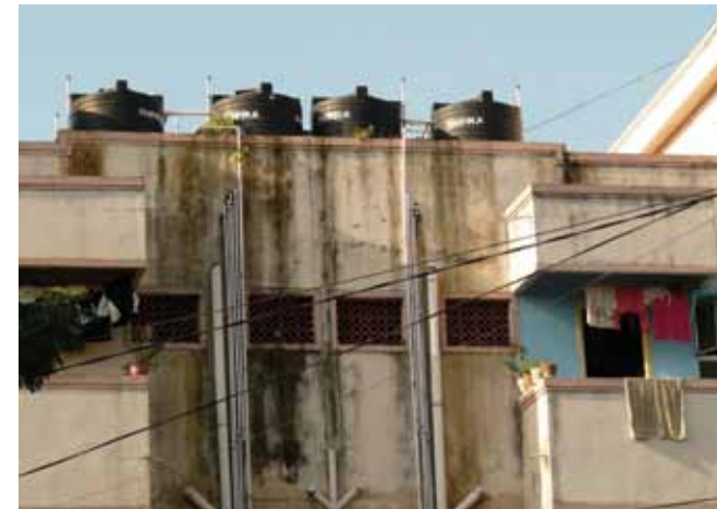
Figure 6: Urban Rainwater Tanks.
