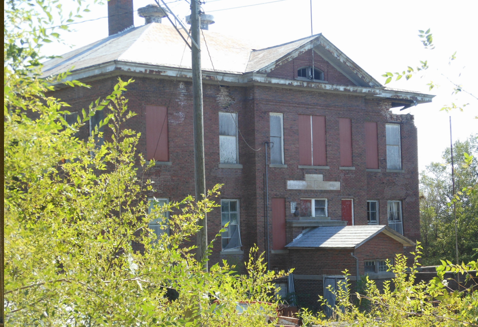
Figure 2. Photo of Former Union, NE Schoolhouse as it Stands Today (Photo by Gibson, August 2012)
