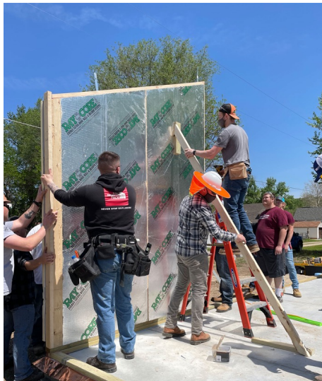
Fig 8 (top): The studio's first project, created with the Mattie Rhodes Center by the 2018-19 studio and built by the non-profit Emerging Builders. The studio designed the home, built the wall and roof panels, pre-installed windows, and prefabricated the central core of built-in cabinets and closets. The home's HVAC system runs in a simple straight line above the central core.
