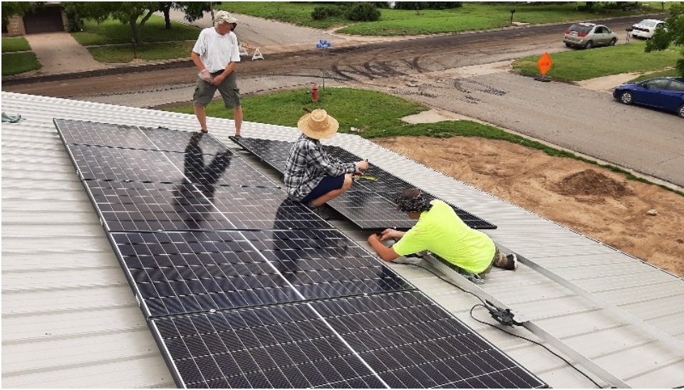
Fig 11: Volunteers from Manhattan-based Flint Hills Renewable Energy and Efficiency Cooperative installed the photovoltaic array in St. John. Solar installations like this one are more affordable every year, with prices falling below $10k for a system of this size; in the meantime, the efficiency and output of PVs is rising. In sum, net zero is more affordable than ever for small homes like those designed and built by the Net Positive Studio.
