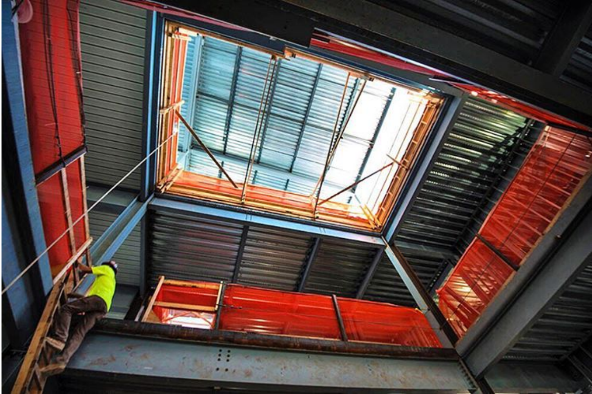
A worker accessing an upper level in the new Regnier Hall. -Photo by Tom Leopold
